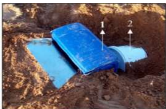
Fig (4) Trough used for collecting rainwater runoff.
